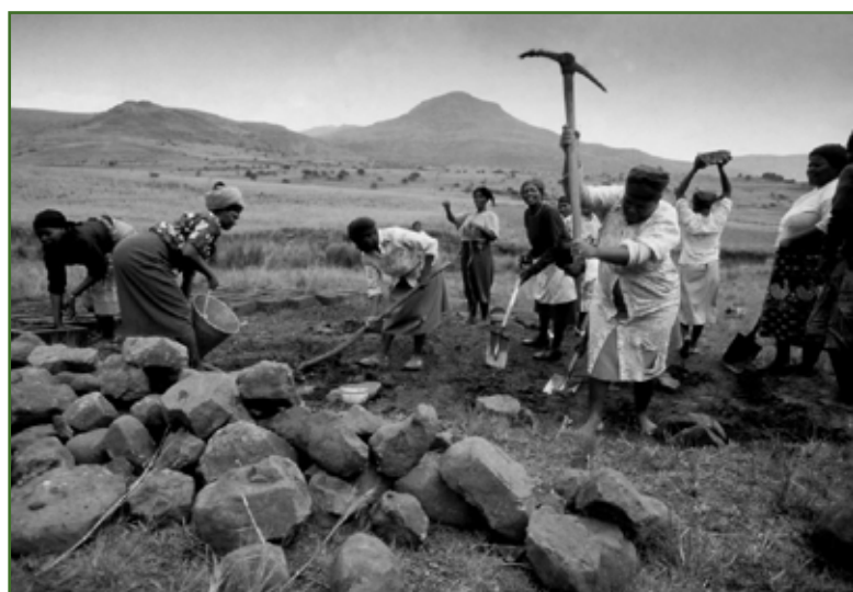
Above: 1988 BETANI VILLAGE, TRANSKEI HOMELAND, The women of Betani sing as they make bricks to make a pumphouse that will hold a pump donated by a concerned corporation. The pump was sent to pump clean water from a river to the village at the top of the hill.
